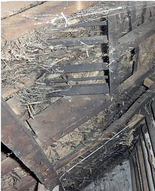
Figure 14: Botley, Sooted window within roof space
